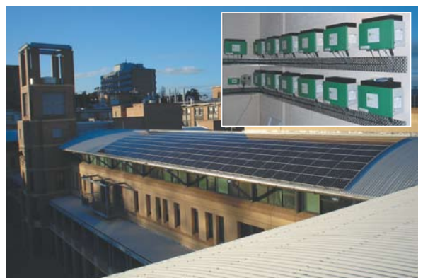
Medium sized system using multiple inverters (6)
